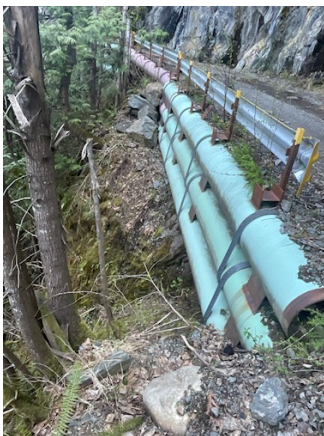
Wall facing with questionable foundation
