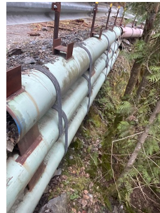
Woods side facing questionable foundation
